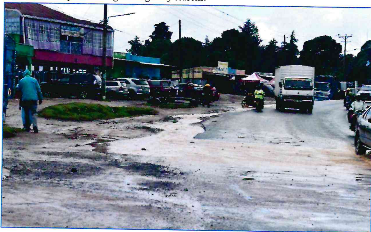
Figure 3 Poor road drainage of municipality roads
