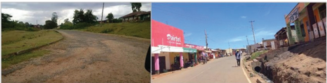
Plate 2 : Left_ Is the Status of roads in Bendera Town. Right_ is a road in Makutano town lacking other road elements.
